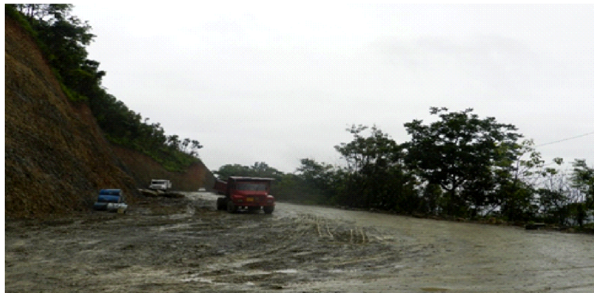
Work Underway on the Road from Champhai to the Border at Zowkhathar
